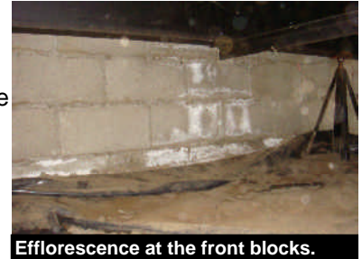
Efflorescence at the front blocks.
