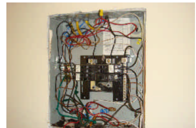
View of the office panel live wire ends
