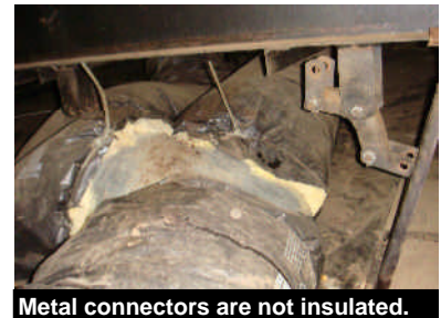
Metal connectors are not insulated.
