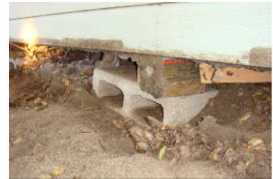
Improper office building support.
