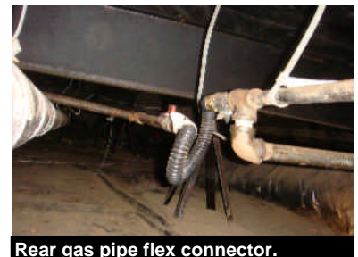
Rear gas pipe flex connector.
