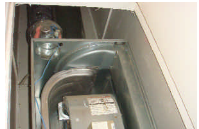
Fresh air ducts at the top of the furnac
