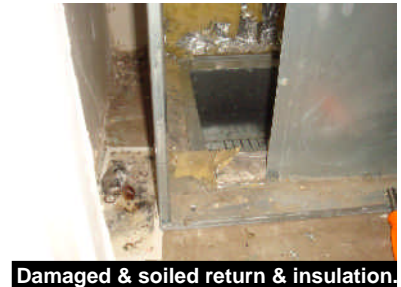
Damaged & soiled return & insulation.
