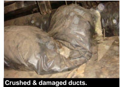
Crushed & damaged ducts.
