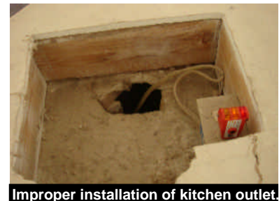
Improper installation of kitchen outlet.
