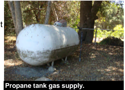
Propane tank gas supply.
