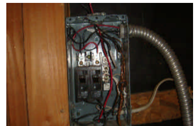
Shed sub panel improper wiring.
