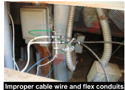
Improper cable wire and flex conduits
