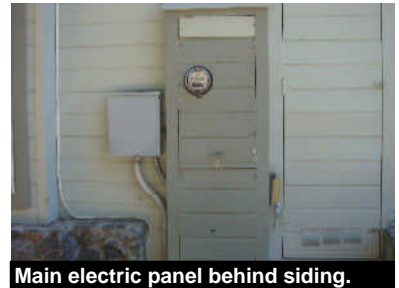
Main electric panel behind siding.
