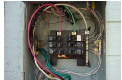
View of the garage sub panel.
