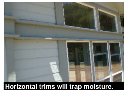
Horizontal trims will trap moisture.
