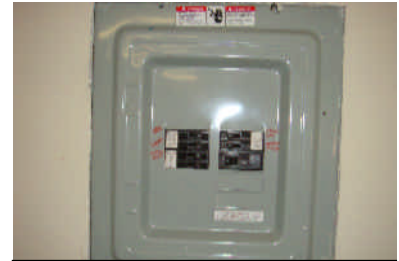
The office panel cover lacking screws
