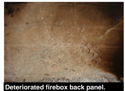
Deteriorated firebox back panel.
