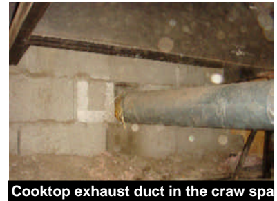
Cooktop exhaust duct in the craw spa
