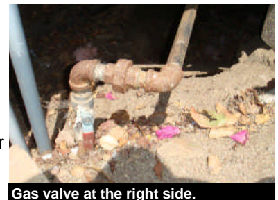
Gas valve at the right side.
