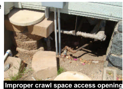
Improper crawl space access opening
