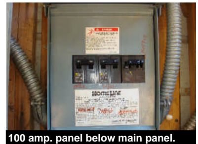
100 amp. panel below main panel.
