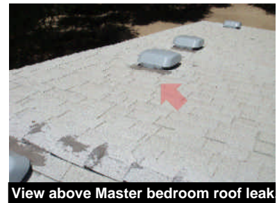
View above Master bedroom roof leak
