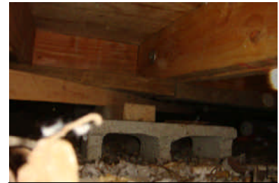
Underside office floor improper support.
