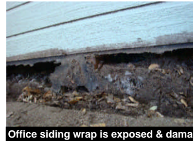
Office siding wrap is exposed & dama
