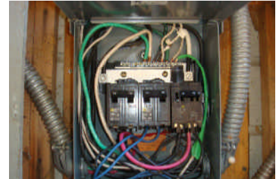
100 amp panel feeding 50 amp discon
