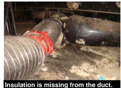
Insulation is missing from the duct.
