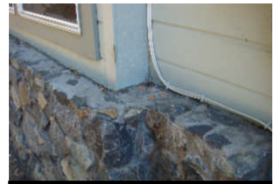
Stone covering the siding improperly.
