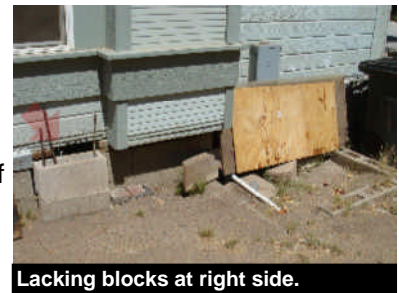
Lacking blocks at right side.
