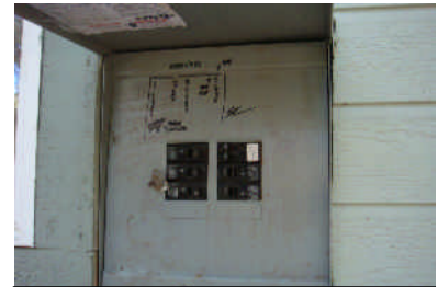
The garage panel cover missing screw
