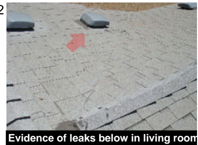
Evidence of leaks below in living room
