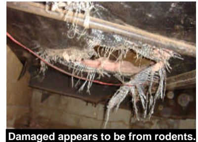
Damaged appears to be from rodents.
