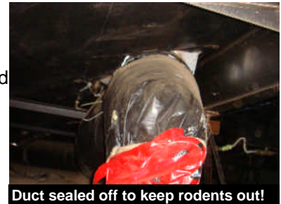
Duct sealed off to keep rodents out!
