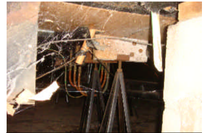
Drain pan & TPRV discharge line.
