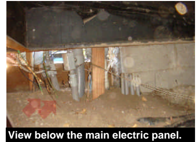
View below the main electric panel.
